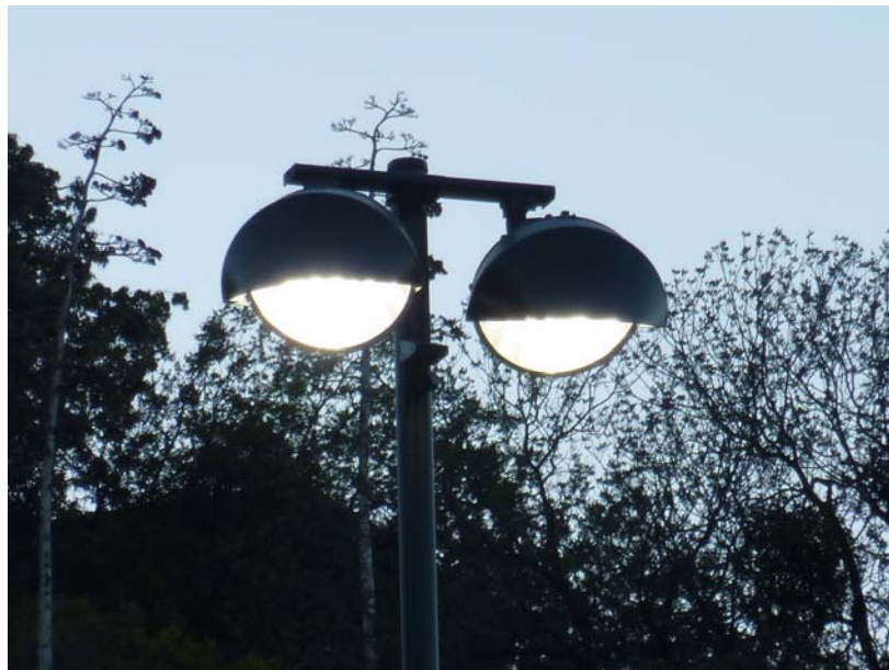
Existing Musco Fixtures
